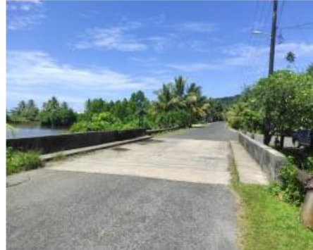
Figure 1.1: Awak Bridge in Pohnpei for replacement.
