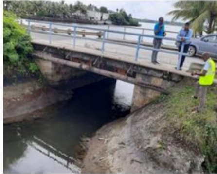
Figure 1.1: Donoch Bridge in Yap for replacement.
