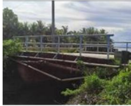
Figure 1.2: Tagaaniyal Bridge in Yap for replacement.
